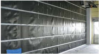
SOUND PROOF, BUS DUCT & CABLING SYSTEM
