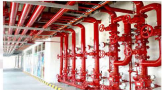
FIRE FIGHTING SYSTEM
