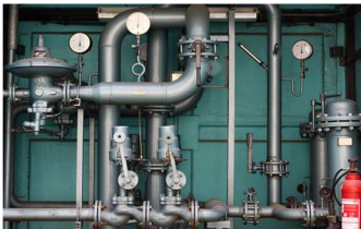
FUEL SYSTEM (WITH ALL PARTS)
